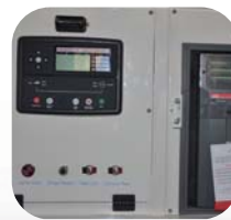
Control Panel & MCB
